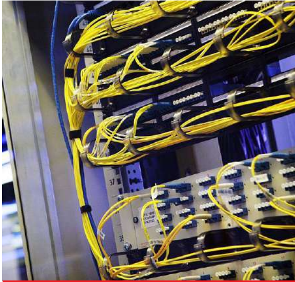
Figure 9: Fiber Optic Cables
