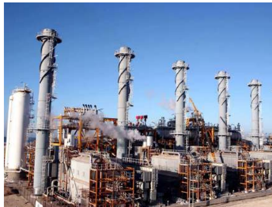
Figure 11: KPC Bulk LPG Storage Handling
