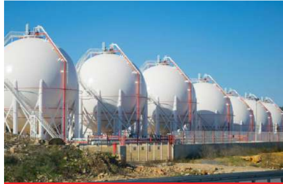
Figure 11: KPC Bulk LPG Storage Handling
