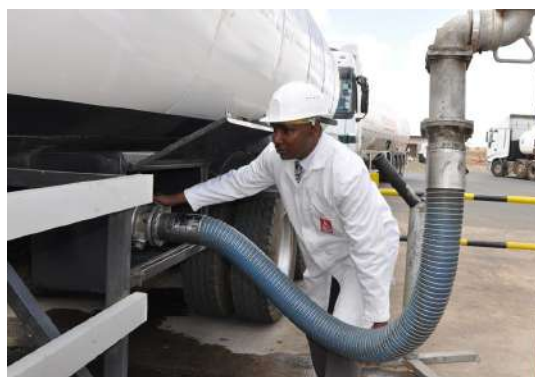
Figure 7: KPC Bottom Truck Loading Facility
