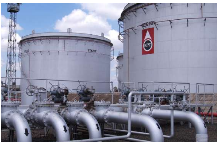
Figure 1: KPC pipeline Storage Facilities
